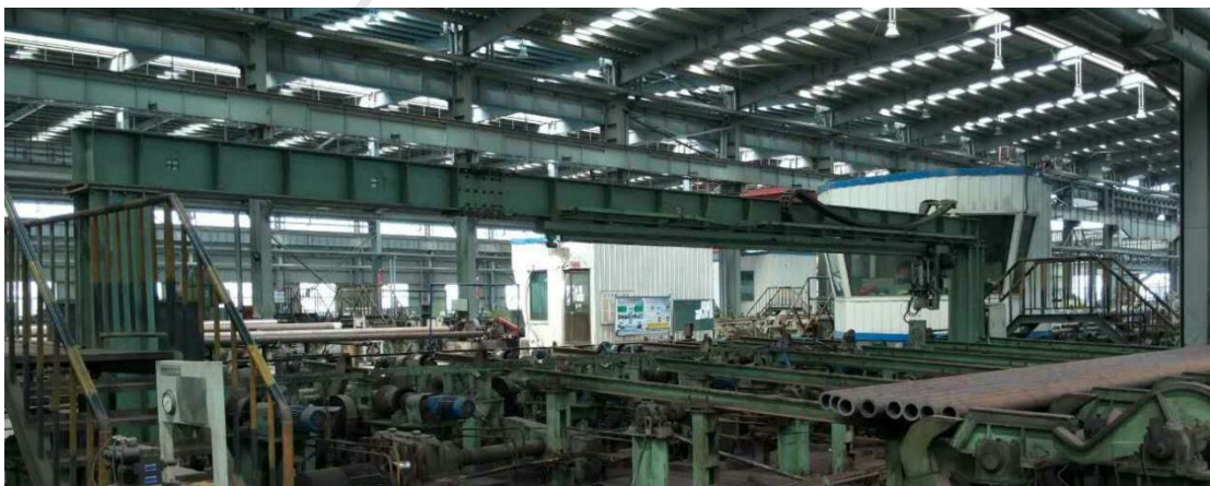
Online automatic marking equipment
