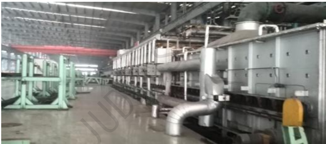
Heat treatment equipment (normalizing furnace)
