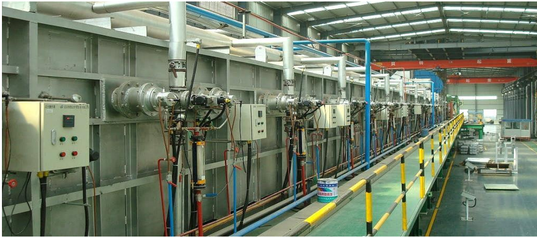
Heat treatment equipment (annealing furnace)
